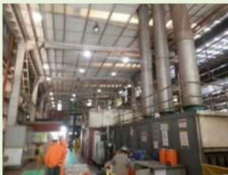
Vista Interna do Shot Blasting I
