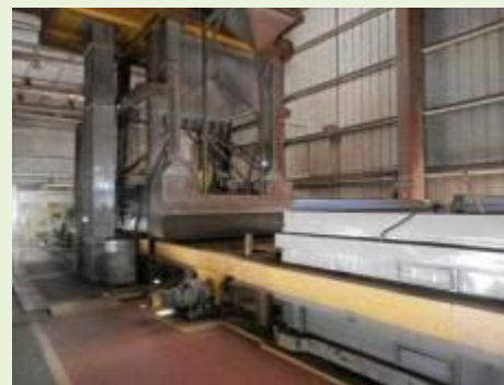
Vista Interna do Shot Blasting
