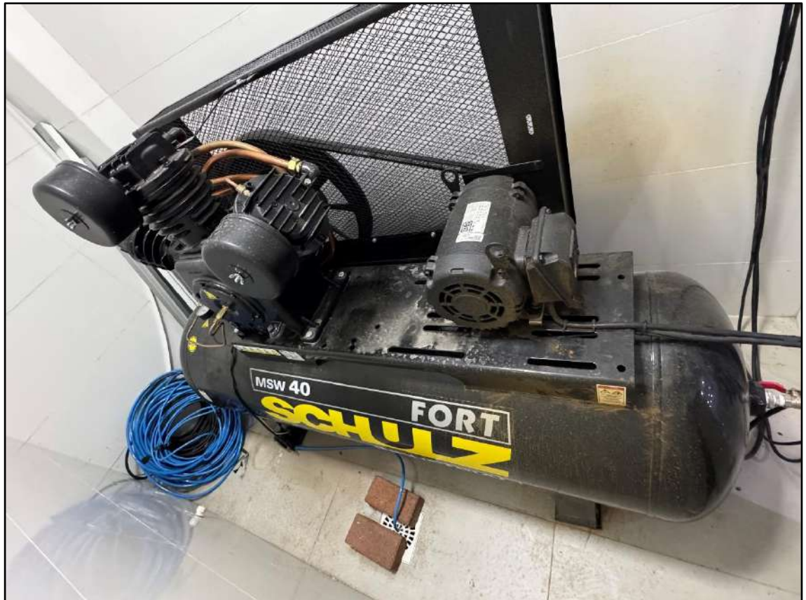
ITEM 046 - COMPRESSOR SCHULTZ MSW 40
